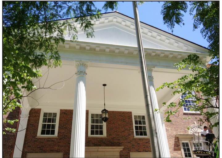
The Award acknowledges restoration of the slate roof, original wood windows and exterior masonry.
