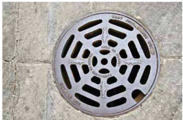
Storm sewer drain in Oak Park. Source: Jim Watkins
