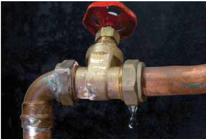
Household leak. Image courtesy of iStockphoto.com.
