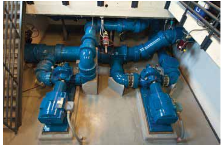
Variable Speed Pumps; Used for soft start and stops reducing water hammer and consistent flows and pressures. Source: Oak Park.
