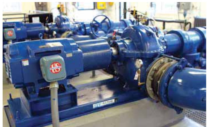
Variable Speed Pumps at the Oak Park Central Pumping Station. Source: Oak Park.
